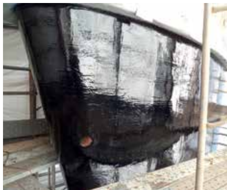
Above: Belzona cavitation protection system application to a Naval vessel in Japan
