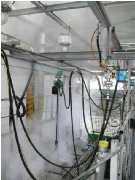
J D Neuhaus air operated hoist in operation for precise handling of pressure injection head during tank cleaning operation.
