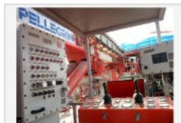
Hazardous Area Crane Control Systems
